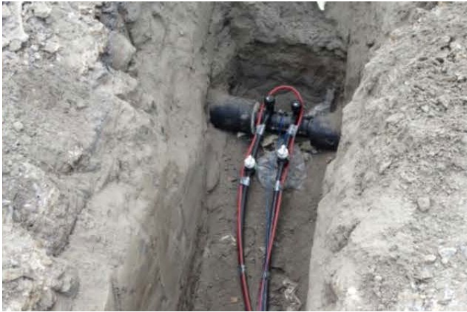
Lateral joining loop with red PEX pipe heating loop
