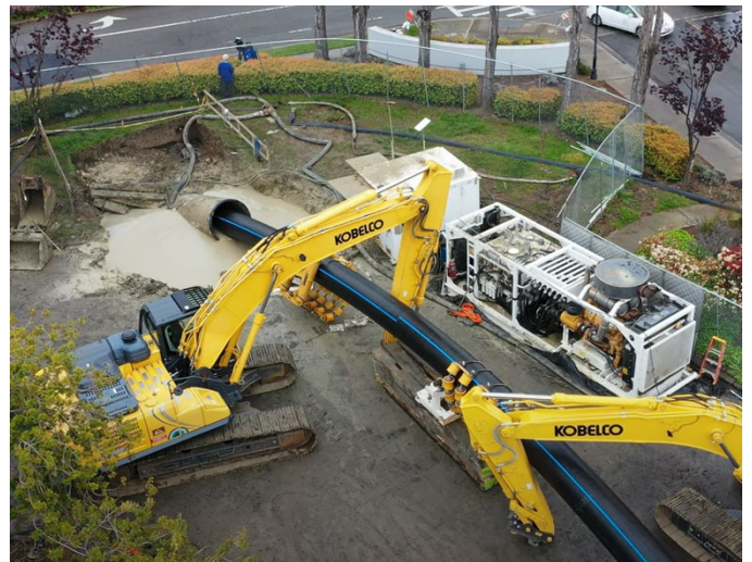
Figure 2: Fused 32-inch diameter PE4710 pipe string on rollers being pulled to the borehole
