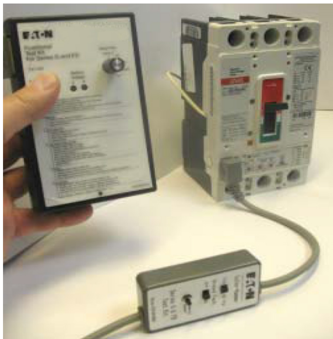
Figure 8. Testing a Circuit Breaker.
