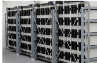
Energy Storage System
