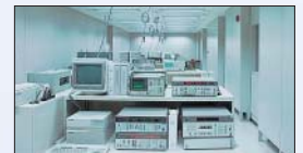
Temperature- and humidity-controlled calibration room
