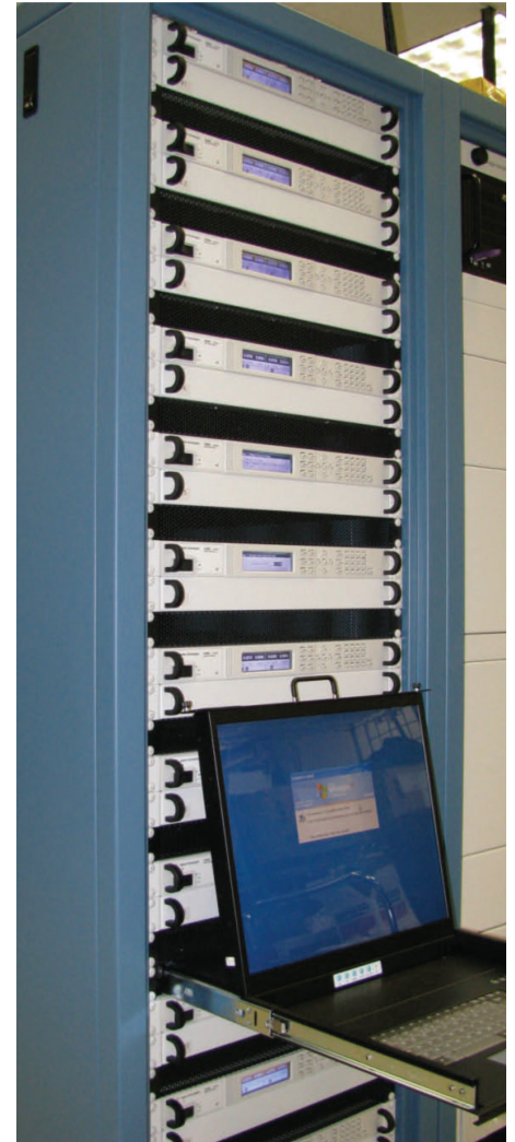
Figure 6. Custom turnkey system
