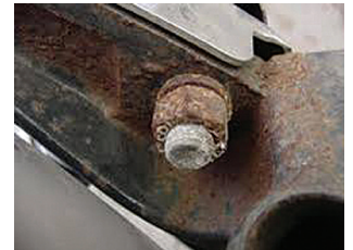
Figure 12. Rusty Bolts can cause PIM.
