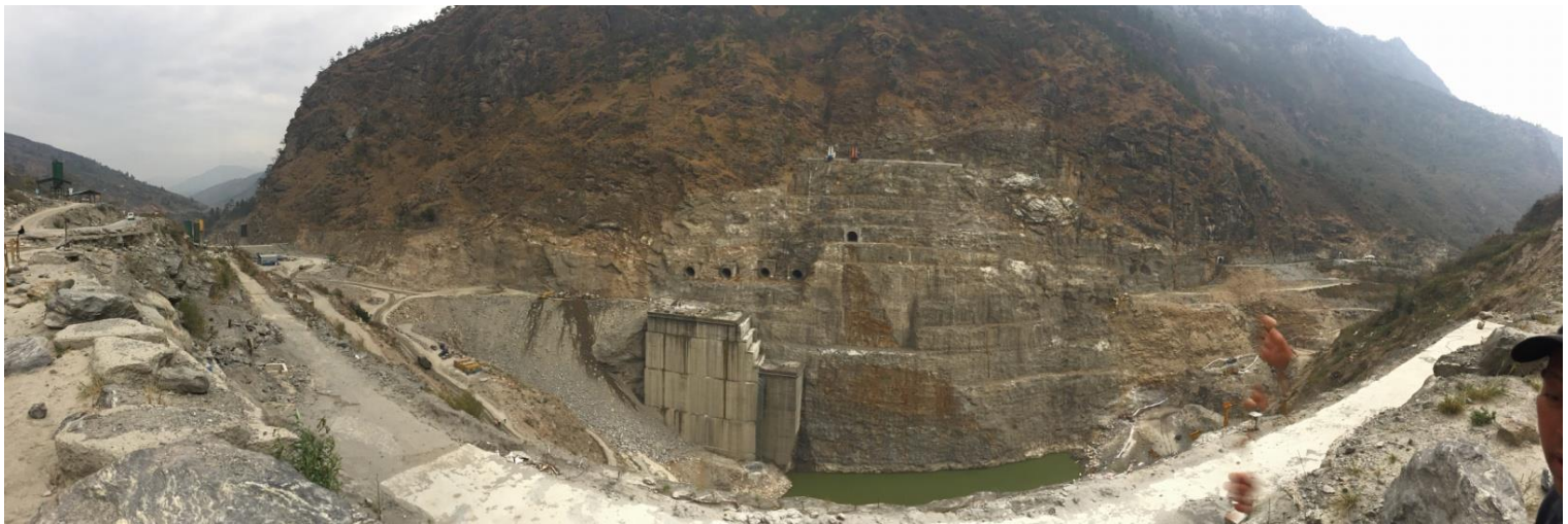
Fig. 65) A panoramic view of the Punatsangchhu-1 Hydroelectric plant construction site as seen during a visit on 29-03-2017. The scale is hard to convey in this image, the holes in the mountain can comfortably fit two cement trucks side by side. Image source: Author.
