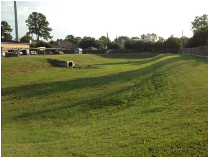
Figure 13: Dry detention pond (Suckers, 2015)
