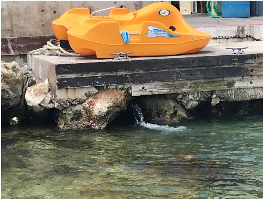
Figure 56. Kim Sha Beach water testing site with a hotel pipe discharging gray-water visible underneath the dock.
