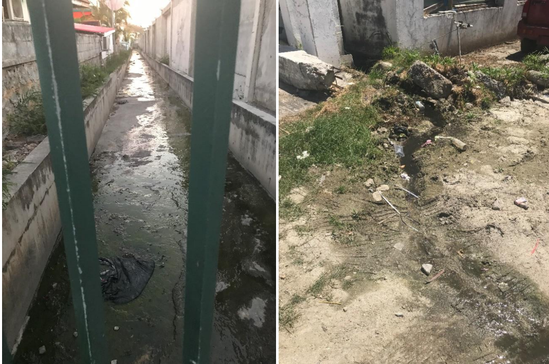
Figure 45. Sewage in a storm gutter and flowing from a house in Cole Bay, 2019.
