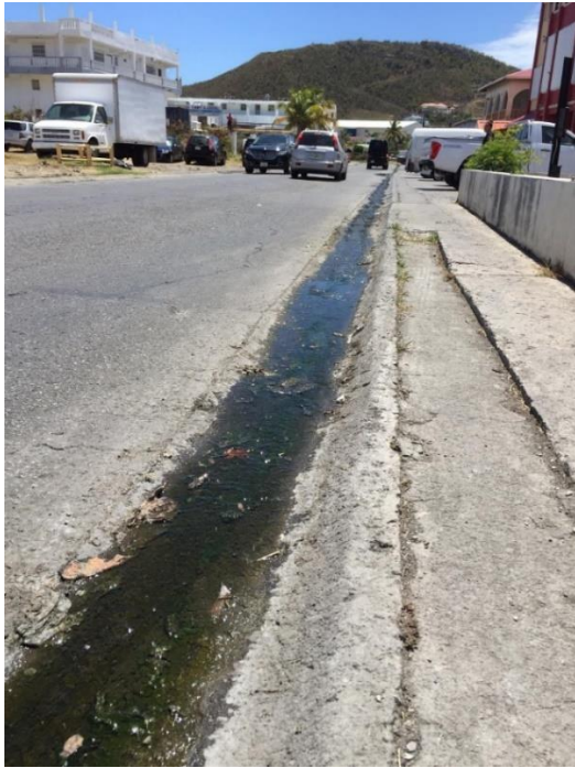
Figure 16. Storm gutter with sewage in Cole Bay, May 2019.
