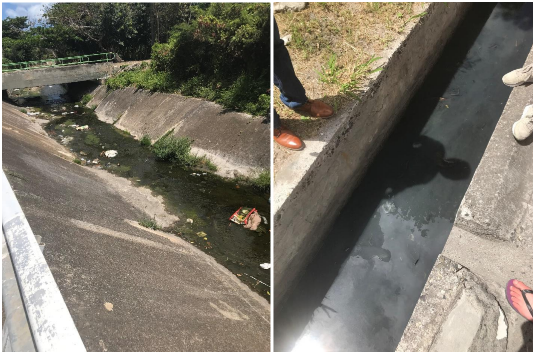
Figure 46. Sewage in storm gutters in Cul-de-Sac and Cole Bay, St. Maarten, 2019.
