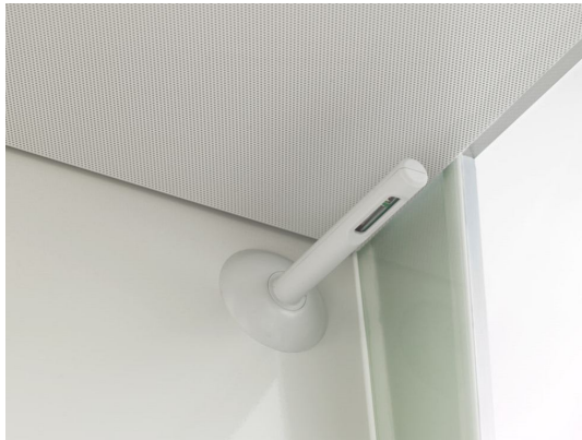
Picture 9. Down flow indicator
