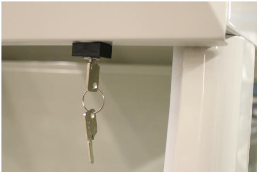
Picture 4. Key switch connects cabinets main power on or off.
