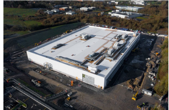
Construction is underway at our new state-of-the-art manufacturing plant in Limerick, Ireland. The new facility is designed for LEED Platinum status.
