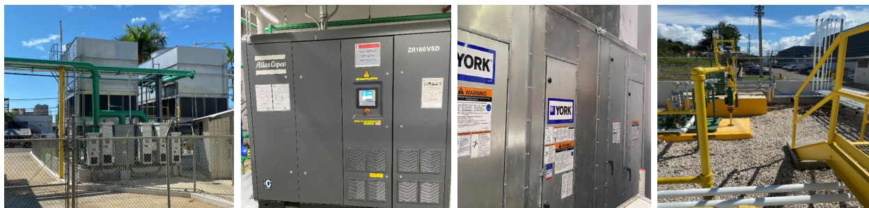
Energy conservation projects at our Puerto Rico manufacturing plant in 2019 included installation of a new cooling tower system which is integrated into the building management system, variable speed drive air compressor, clean room air handling unit and liquefied petroleum gas vaporizer for the cogeneration plant.
