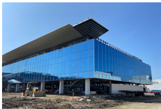
In 2019, construction started on our campus expansion project. The new state-of-the-art “Dream Big Complex,” which is planned for LEED certification, will house R&D laboratories and administrative offices.
