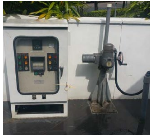
The wastewater monitoring system at our Singapore manufacturing plant ensures water discharged from the site meets stringent Singapore NEWater plant receiving parameters.
