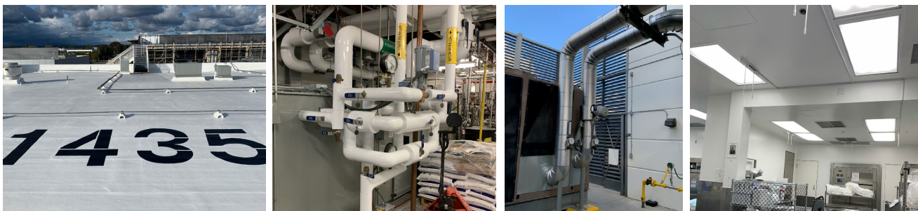
New roof coating, insulation and lighting installed at our Irvine manufacturing plant in 2019 contribute to incremental energy efficiency improvements at the site.
