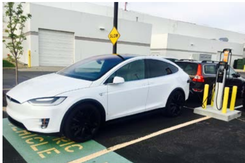
Draper, Utah, Electric Vehicle Charging Stations
