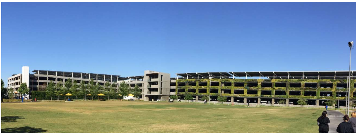
Solar Photovoltaic Panel Electricity System, Top of Parking Structures, Irvine, CA
