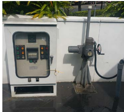
Wastewater Monitoring System
