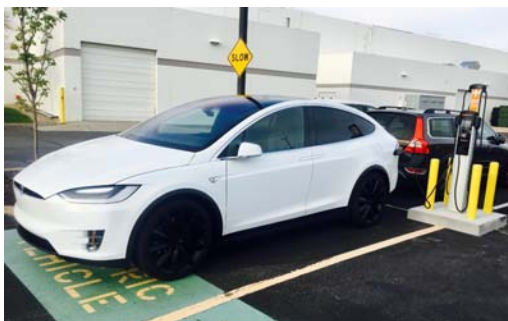
Electric Vehicle Charging Stations
