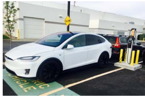
Draper, Utah, Electric Vehicle Charging Stations
