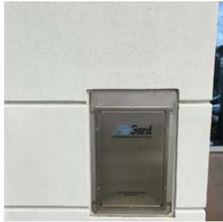
In-Line Filters for Roof Drains & Parking Structures prior to run-off
