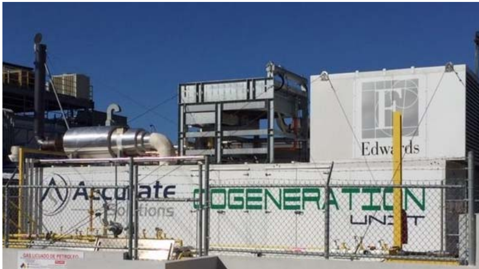
Cogeneration Unit Installed at Añasco, 2017
