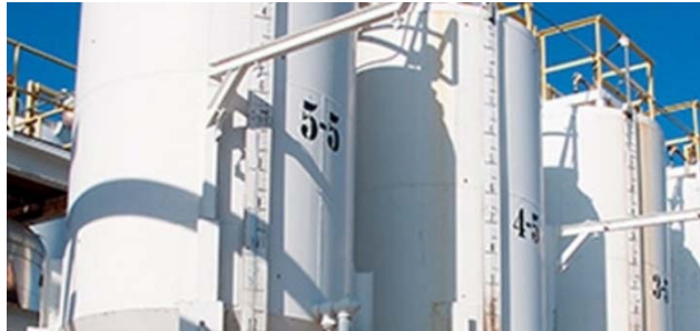
Our Partners' North American Fuels Blending Facility
