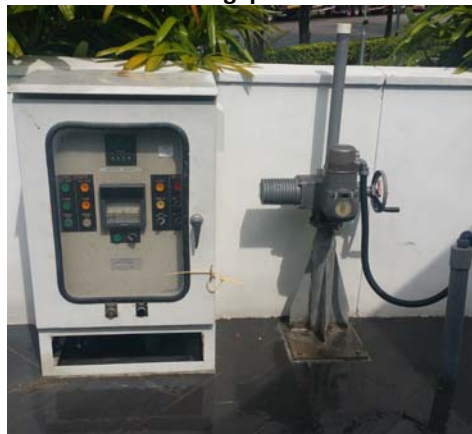
Wastewater Monitoring System
