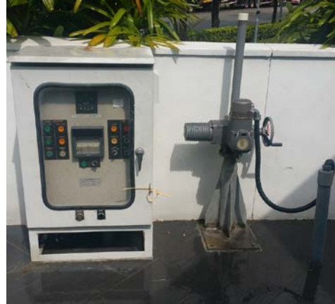
Wastewater Monitoring System
