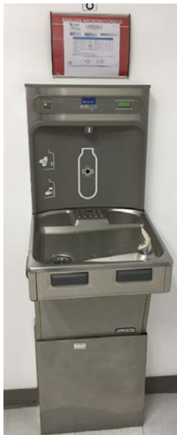
Treated drinking water tested weekly for quality control
