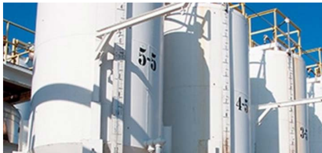
Our Partners’ North American Fuels Blending Facility
