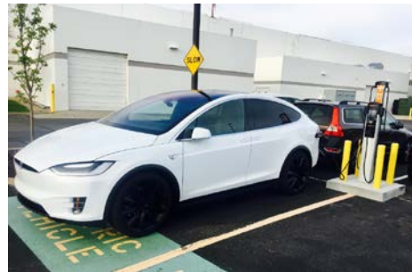
Draper, Utah, Electric Vehicle Charging Stations
