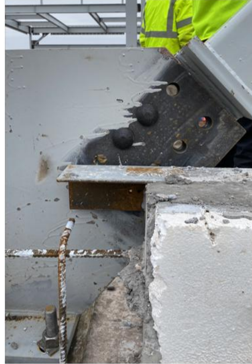
Structural element interference
