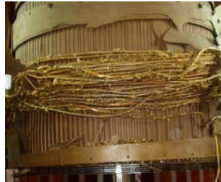
Collapsed tap winding
