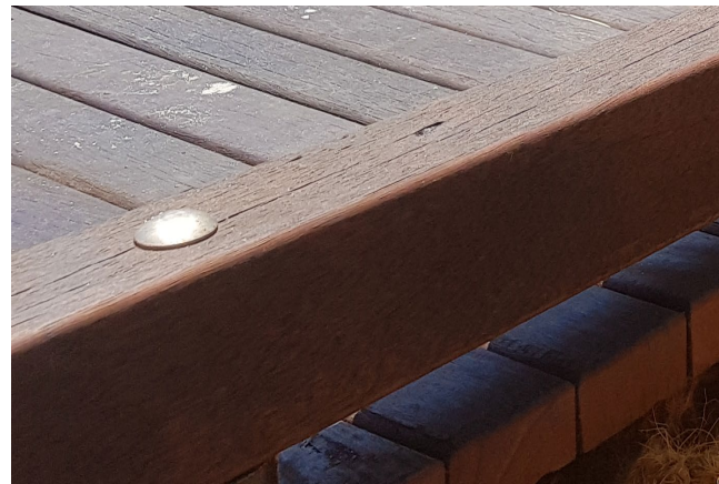
5: Timber deck and edge restraint with stainless steel bolts through timber blocks
