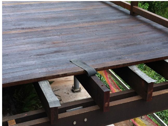
5: Timber deck screwed onto joists with aluminium tape on top of joists
