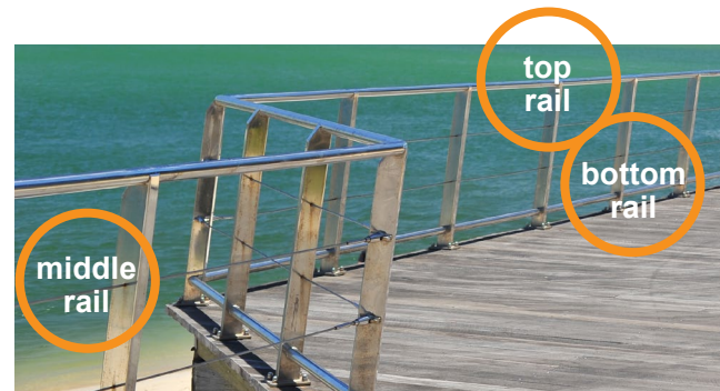
Figure 14: Typical top, middle and bottom rails (for guidance only – site specific design required)
