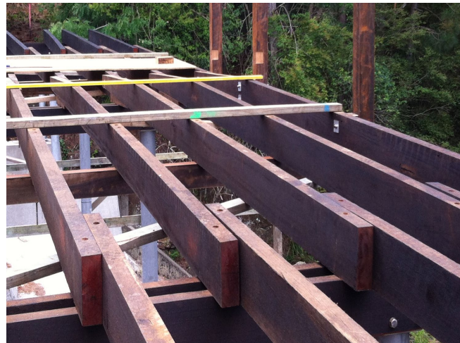
4: Timber joists lapped and fixed onto bearers. Timber posts for balustrade fixed to double bearers
