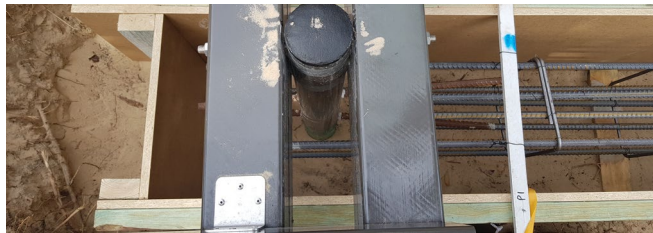
1: Boxing for reinforced concrete strip footings with FRP headstock (bearers) bolted to HDG core filled concrete screw piles, (coated with marine epoxy)
