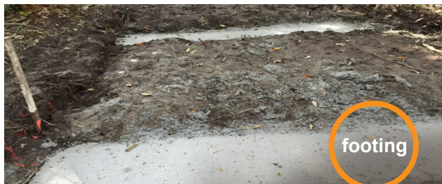
Figure 3: Example – foundation / pad / strip footings (for guidance only – site specific design required)
