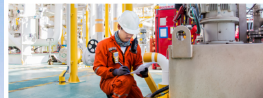
MOTOR CONTROL AND MCCS
