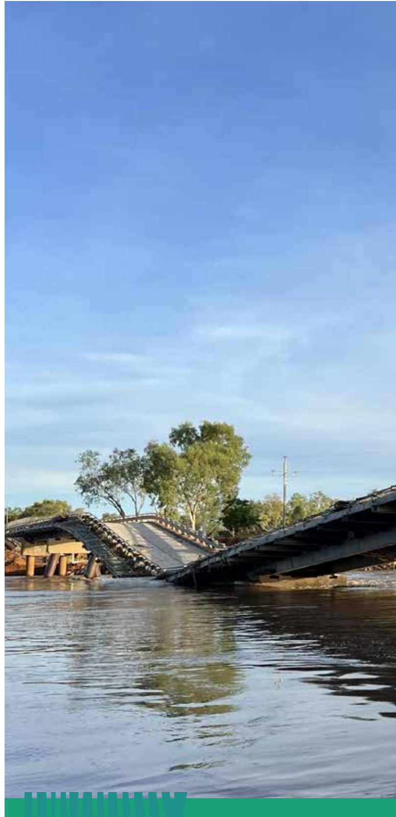
The floods caused the collapse of the Fitzroy River Bridge, which was unusable for close to a year and cut off the only access and transport route to surrounding communities.
