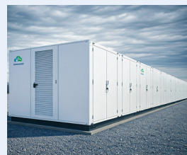
BATTERY ENERGY STORAGE SYSTEM
