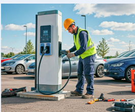
EV CHARGING STATIONS
