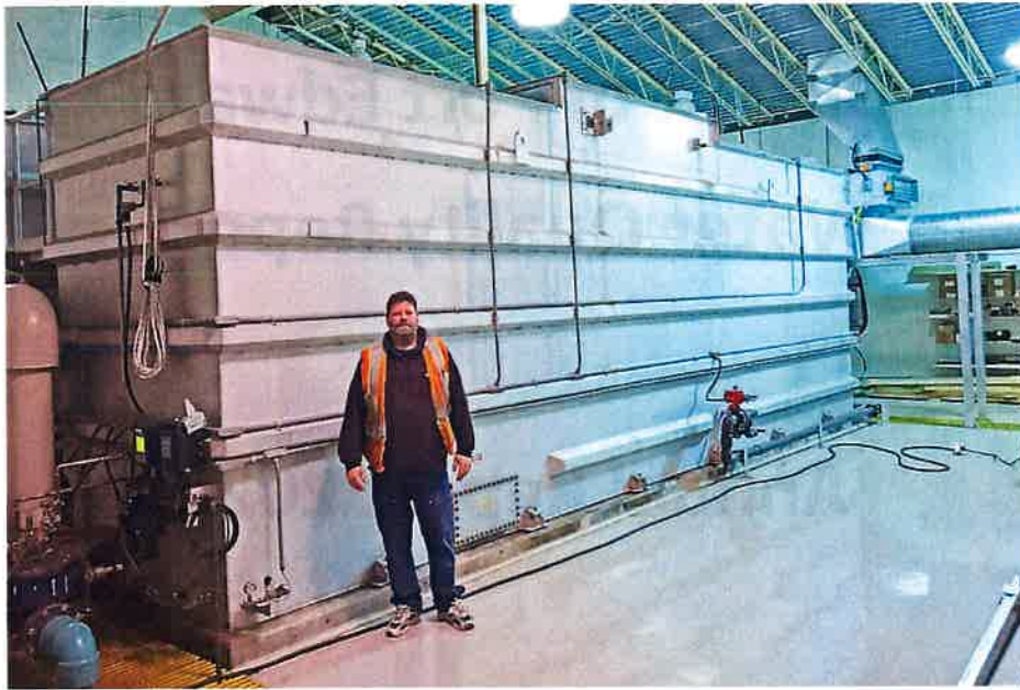
Port Edward Water Treatment Plant with Utility Operator, Scott Duffus
