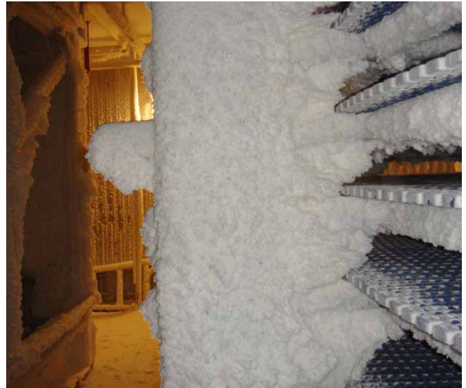
Ice buildup blocks airflow velocity, reducing system efficiency.
