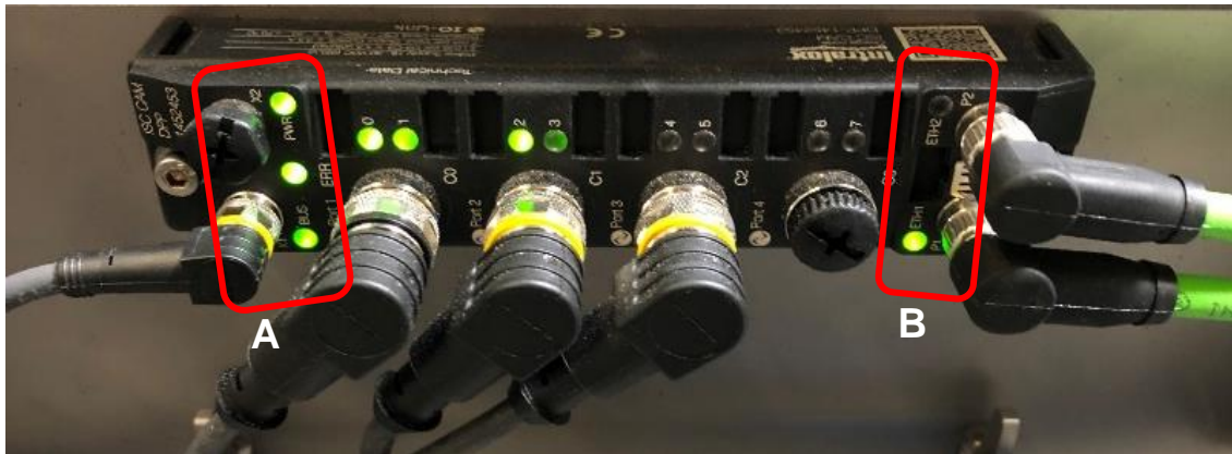
Verify power status
