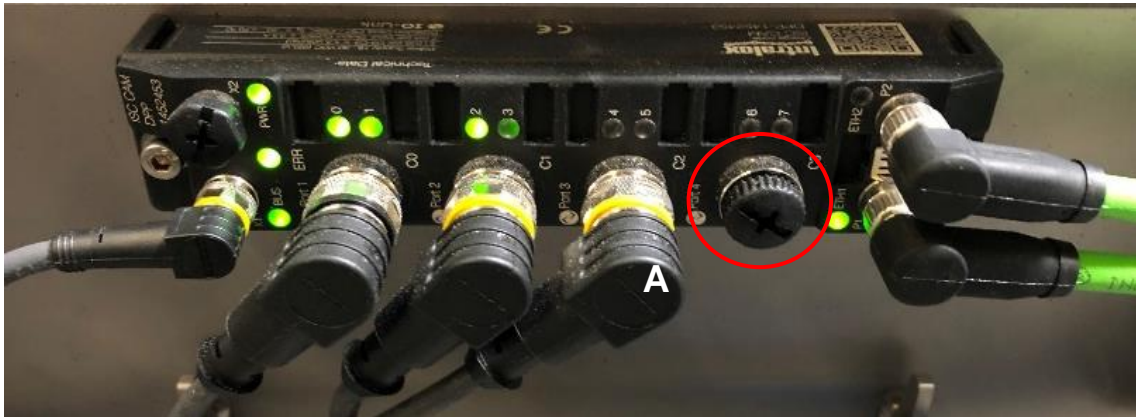
C3 Port for Hardwired signal connections
